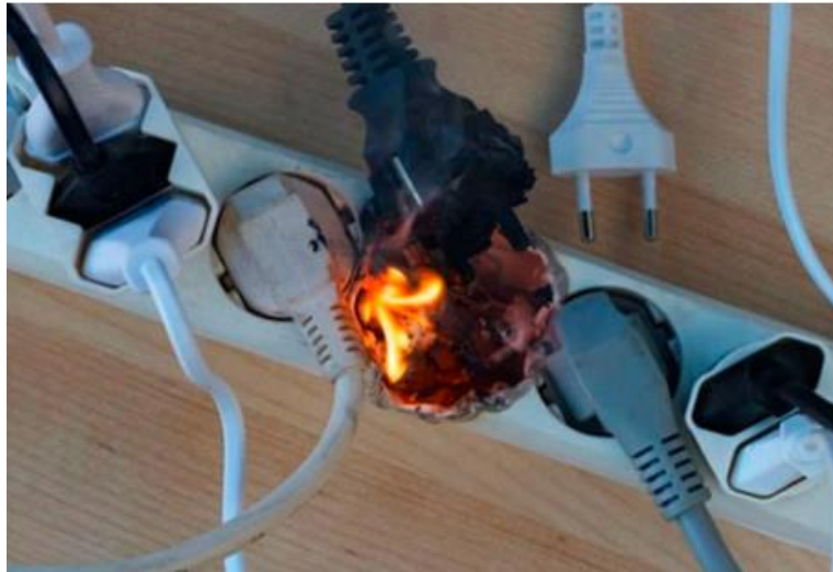
Fig. 1. Electrical equipment the cause of the fire
