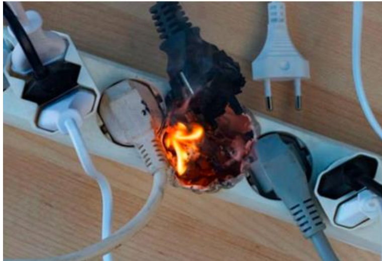
Fig. 1. Electrical equipment the cause of the fire
