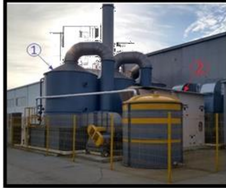
Fig. 3. NMP recovery equipment (1) and air filtration system (2) [source: personal archive]
